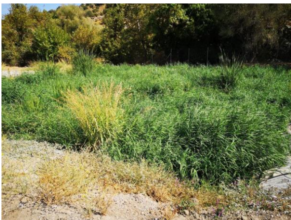
Figure 2. Saturated vertical flow constructed wetland (VF SAT)
